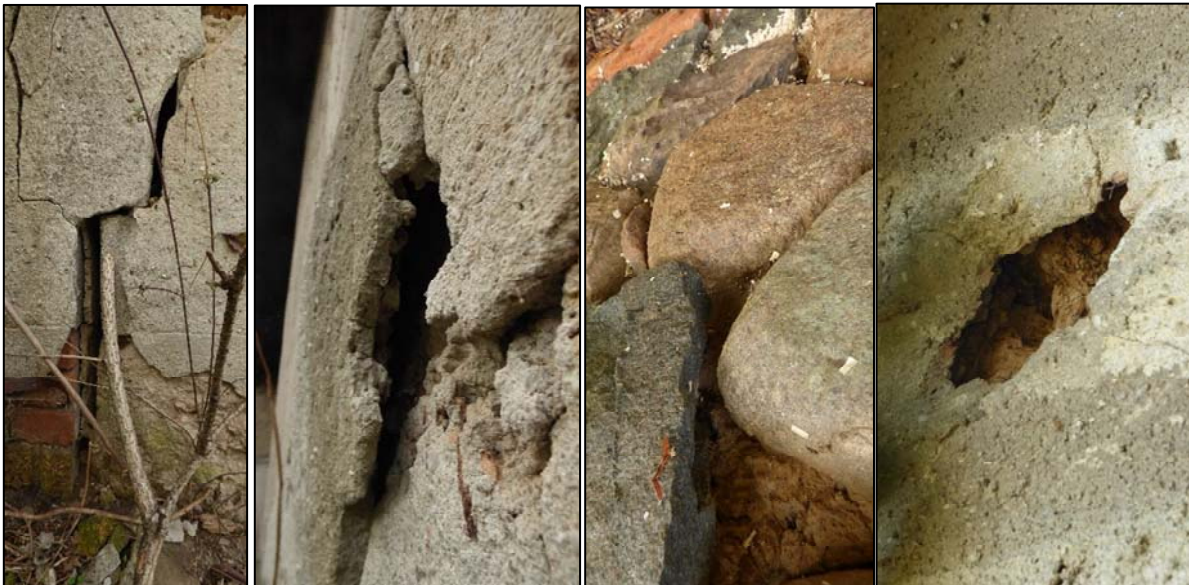
Abb. 9: Risse in Fassade
